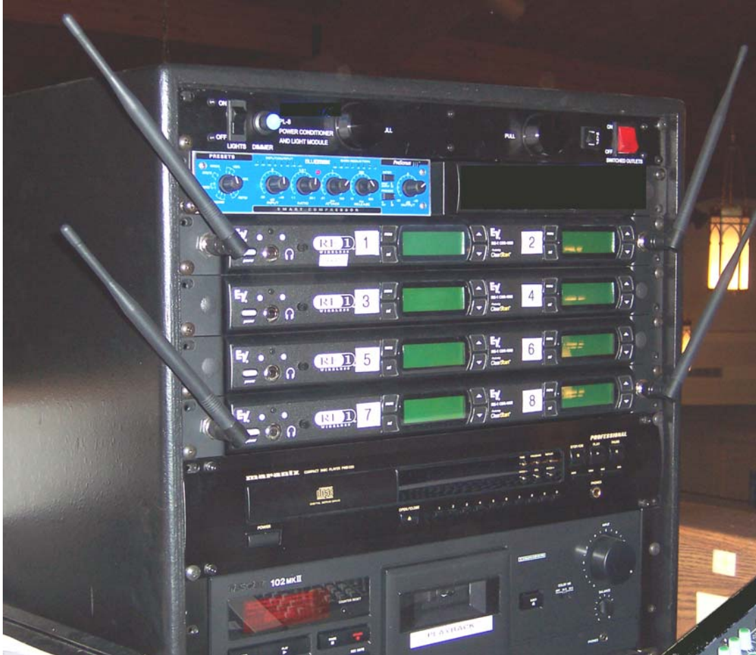
Four EV RE1 Dual Receivers, Racked and Ready to Work
